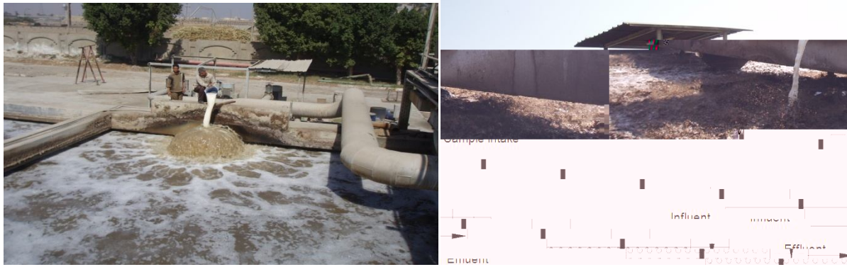
Fig. 1. Photos of the addition of the special microorganisms to the aeration tank
